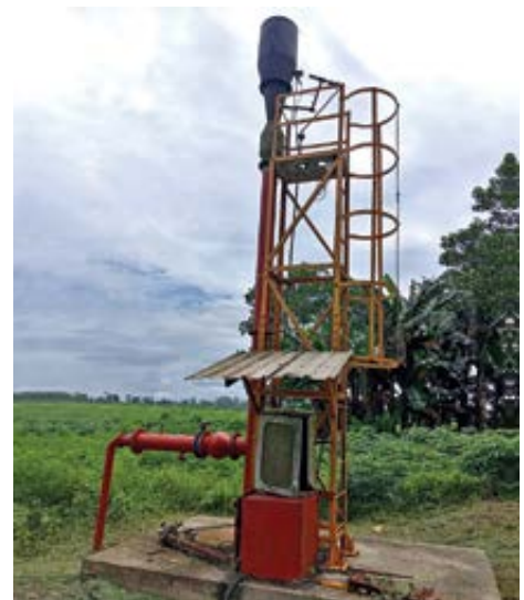
Biogas Flare Stack (Maujaya CPO Mill)
