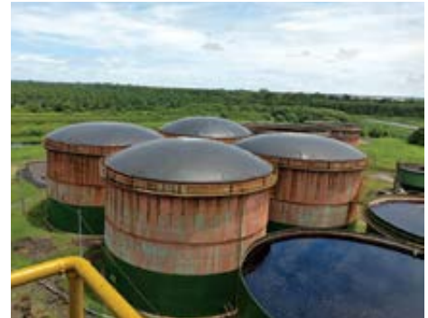
Anaerobic Digester Tanks (Maujaya CPO Mill)
