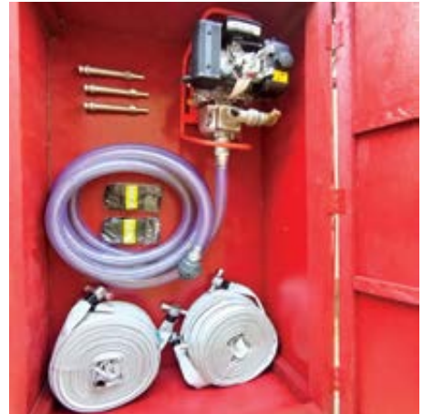
Fire-fighting equipment (Hariyama Plantation)
