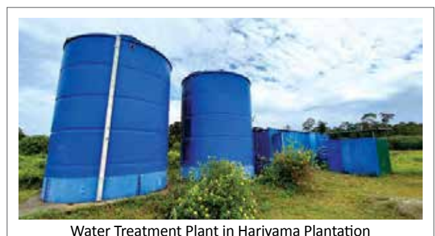
Water Treatment Plant in Hariyama Plantation
