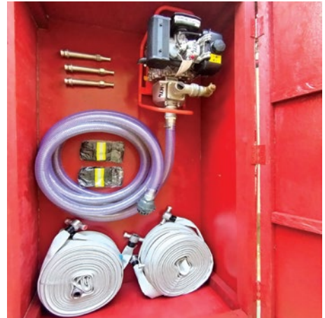
Fire-fighting equipment (Hariyama Plantation)
