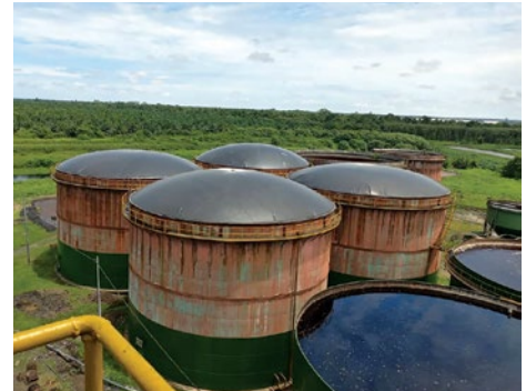
Anaerobic Digester Tanks (Maujaya CPO Mill)
