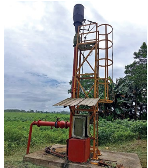
Biogas Flare Stack (Maujaya CPO Mill)
