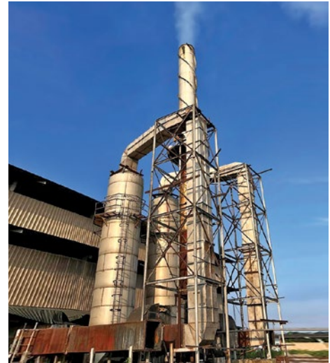
Scrubber system (Hariyama CPO Mill)
