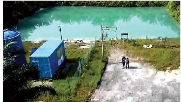
Water Treatment Plant (Sawai Plantation)
